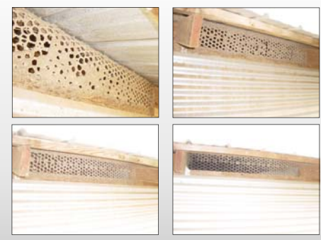
Clogged inlet screens can affect temperature/air quality uniformity
