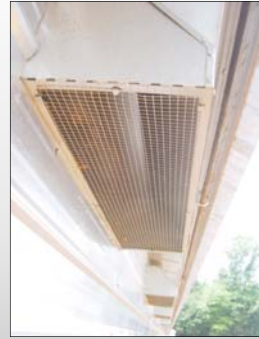
Smaller screen sizes can lead to maintenance issues
