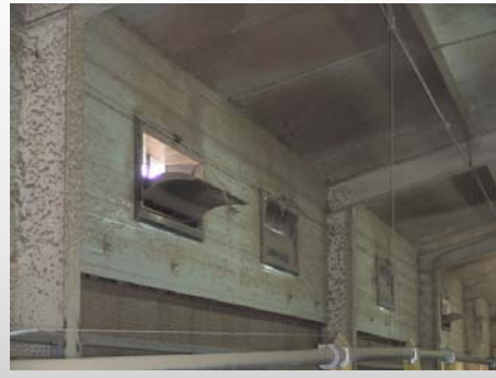
Air flow obstruction in open ceiling house
