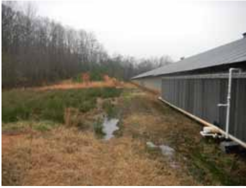
Figure 7. Standing water can lead to foundation problems
