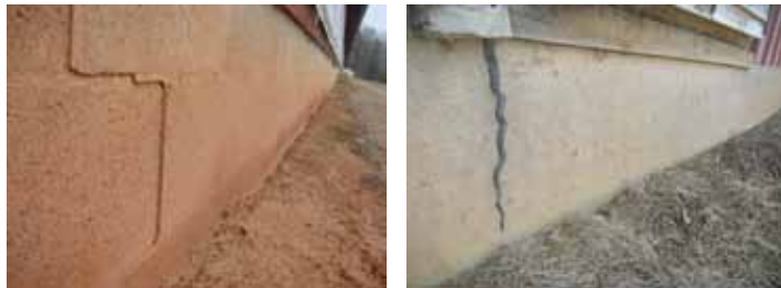
Figure 11. Foundation cracking due to rotation/settling
