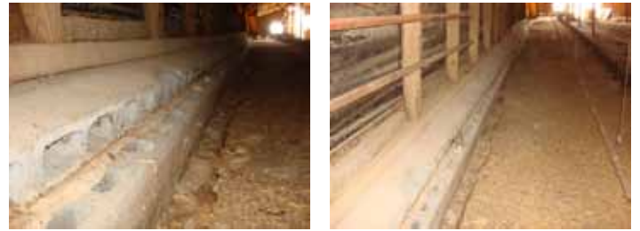
Figure 14. No vertical steel in concrete block side wall
