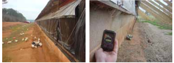
Figure 13. Rotation of concrete block wall foundation
