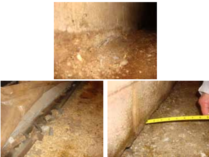
Figure 20. Erosion of block caused by manure
