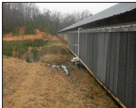
Figure 7. Standing water can lead to foundation problems
