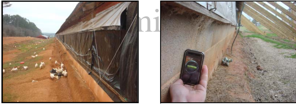
Figure 13. Rotation of concrete block wall foundation
