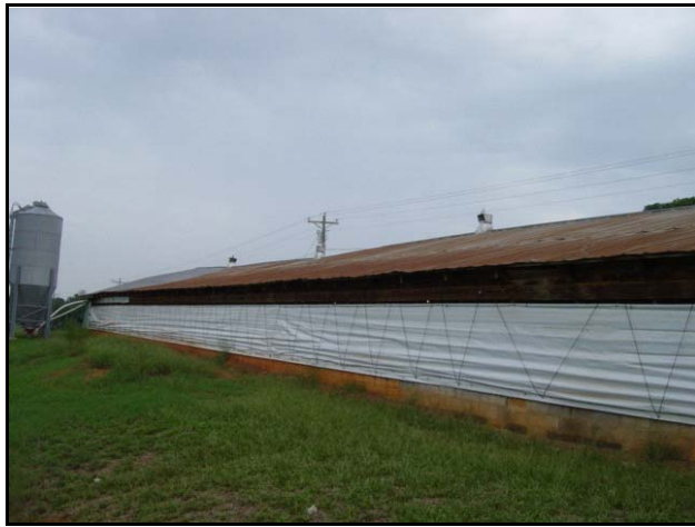
Figure 27. Poultry house with possible truss damage
