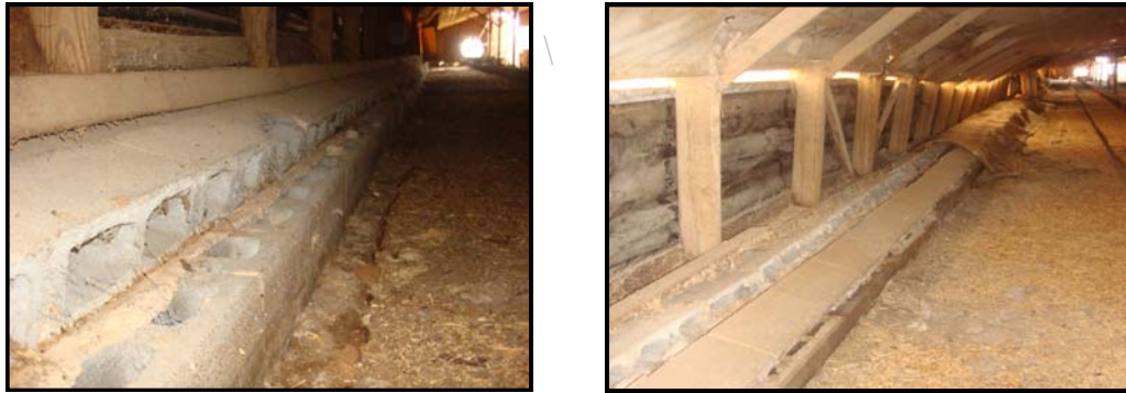
Figure 14. No vertical steel in concrete block side wall.
