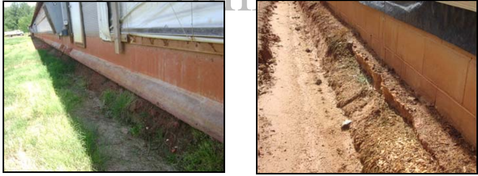
Figure 5. Foundation exposed due to erosion
