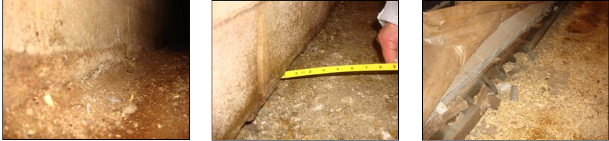
Figure 20. Erosion of block caused by the manure
