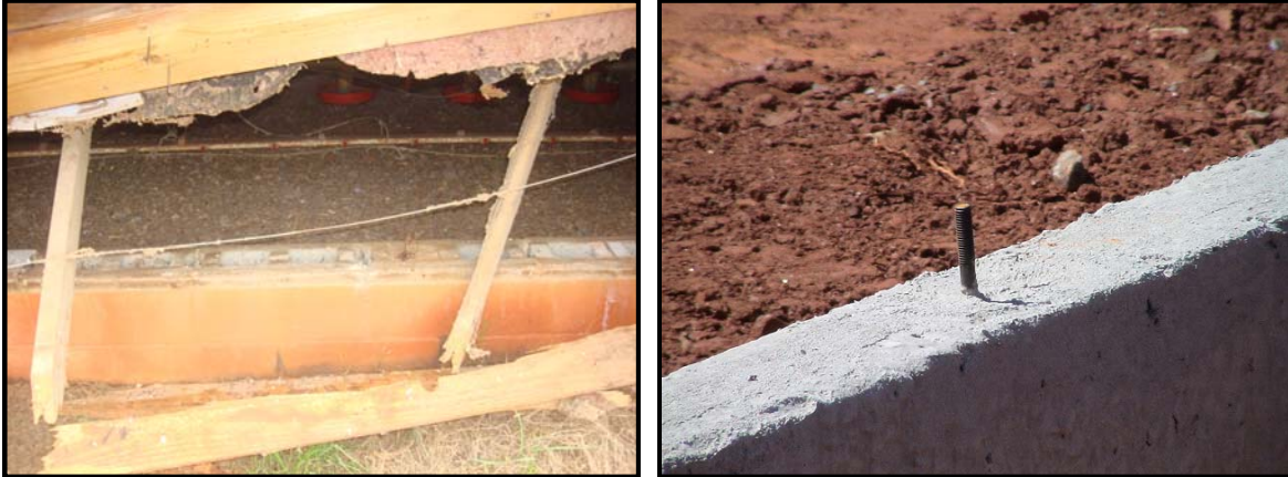
Figure 16. Cores of block should be filled intermittently and J-bolts installed to connect plate to foundation
