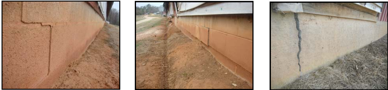
Figure 11. Foundation cracking due to rotation/settling
