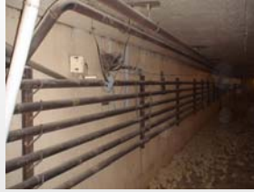
1 1/2" black steel pipe
