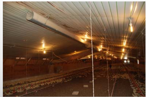
Short duct – with circulation fans
