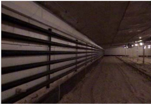
2" black steel pipe
