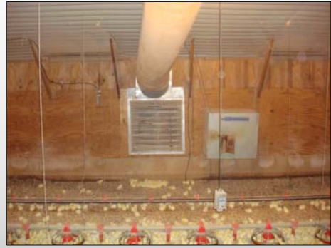
House from air flowing into and out of heating unit
