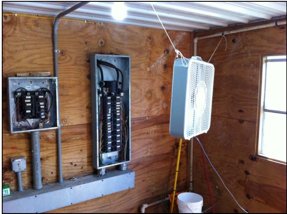
Figure 2. Fan being used to cool overheated circuit breaker.
