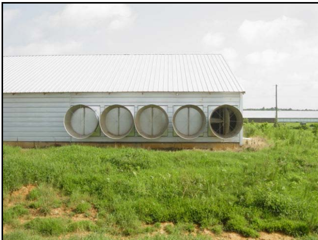
Figure 3. Tunnel fans in side wall starting at end wall.
