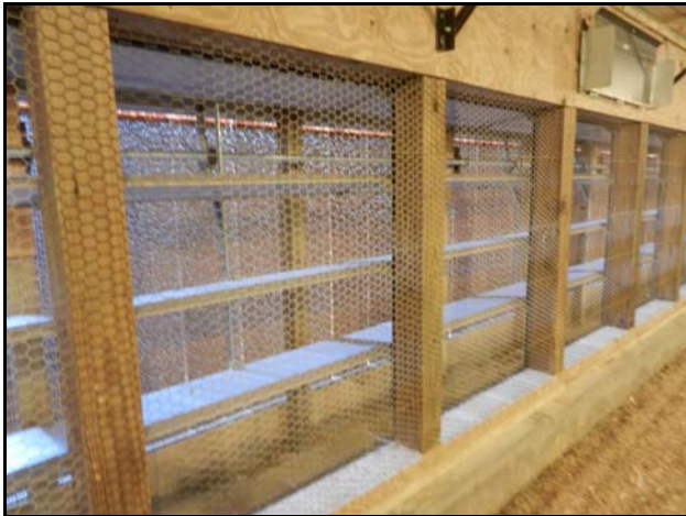
Figure 5. Tunnel inlet shutter.
