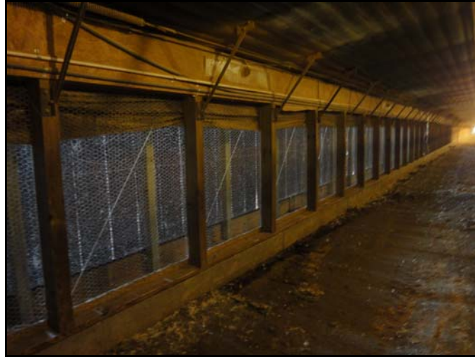
Figure 14. 124' X 6' tunnel inlet curtain opening.
