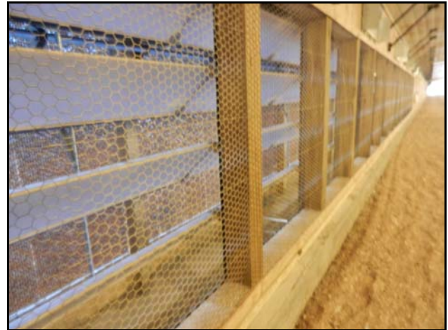
Figure 6. Tunnel inlet shutter partially closed.
