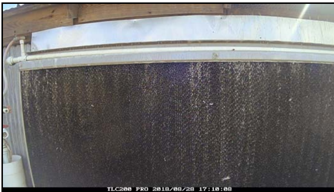
Figure 4. Evaporative cooling pad at 5:10 pm - Day 1 (temperature only)
