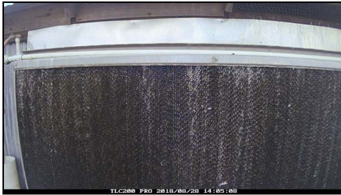
Figure 2. Evaporative cooling pad at 2:05 pm - Day 1 (temperature only)
