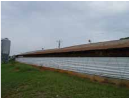
Figure 27. Poultry house with possible truss damage
