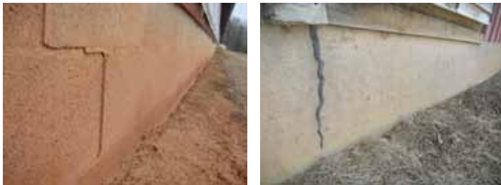
Figure 11. Foundation cracking due to rotation/settling
