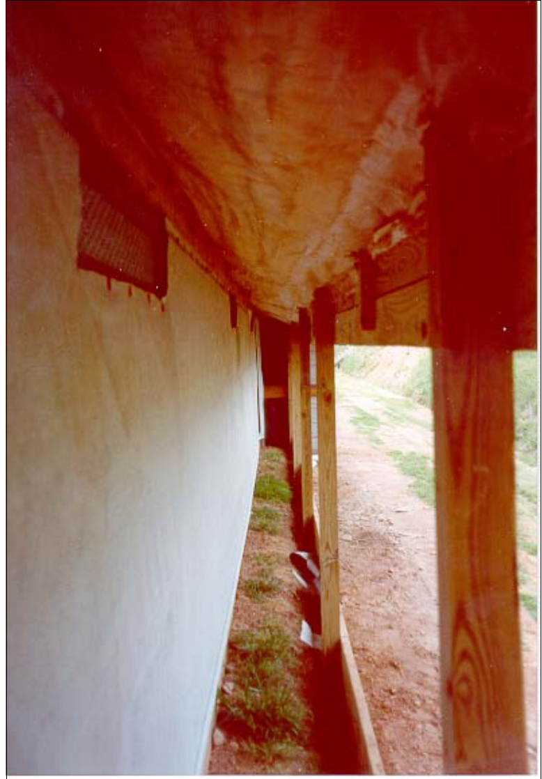
Figure 5. Evaporative cooling pad structure with “dropped ceiling”
