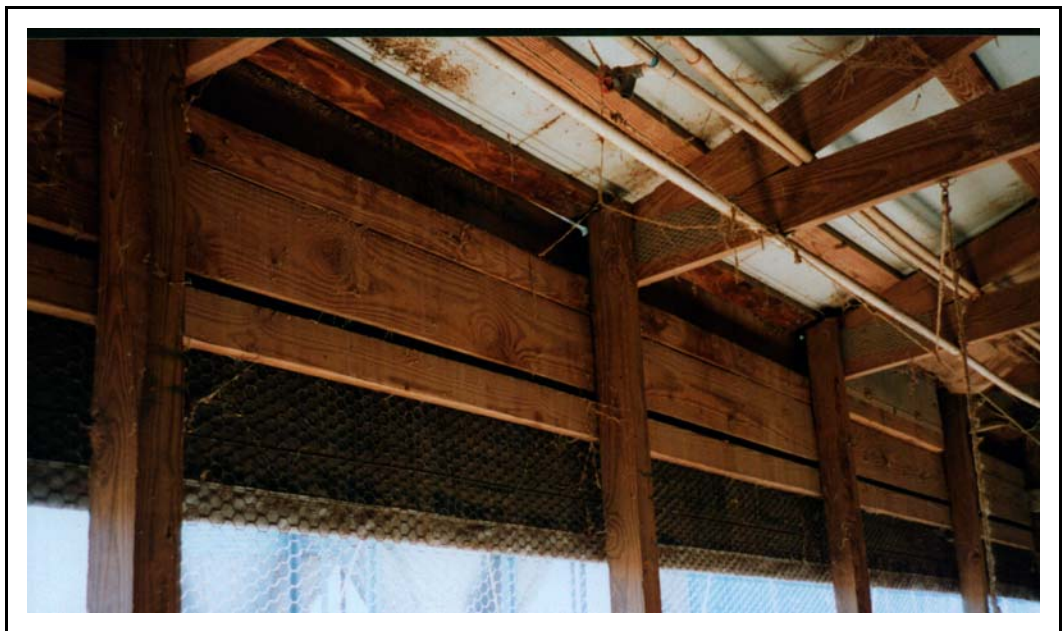
Figure 1. Cracks in top of side wall
