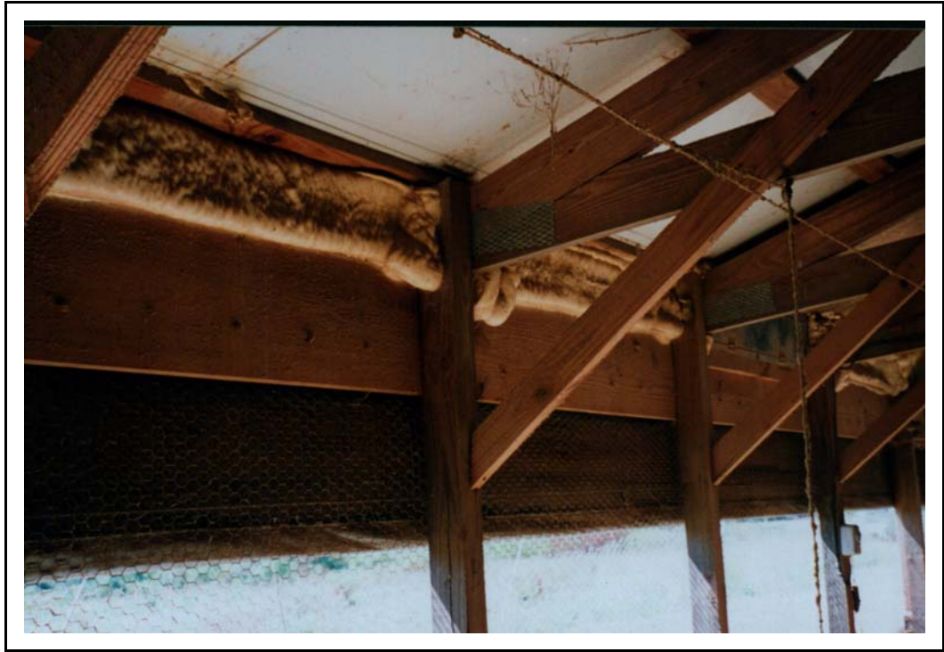
Figure 2. Side wall with sealed cracks
