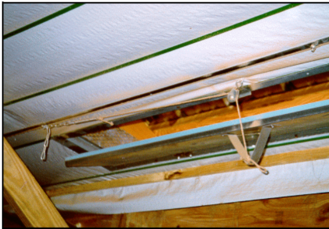
Figure 1. Ceiling inlet with steel banding strip
