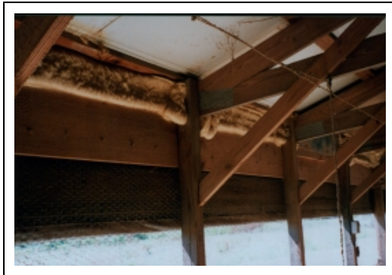
Figure 2. Side wall with sealed cracks
