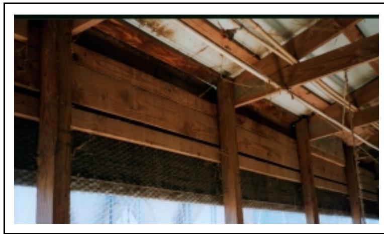
Figure 1. Cracks in top of side wall
