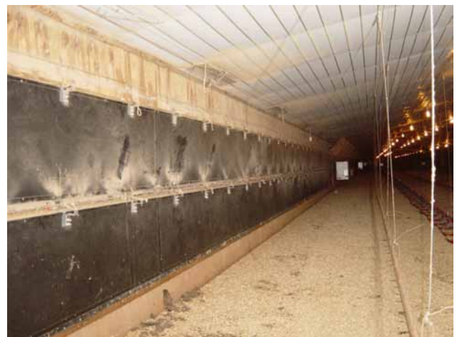
Figure 2. Insulated Tunnel Doors
