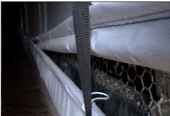
Figure 1. Pocket with electrical conduit
