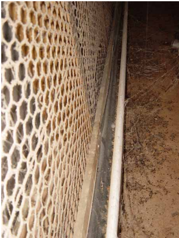
Figure 3. Tunnel curtain pocket
