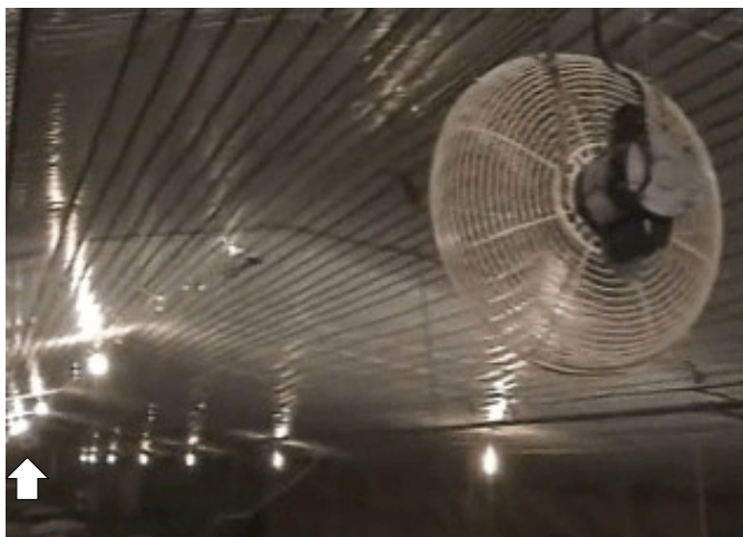
Figure 2. Ceiling circulation fans (arrow points out second circulation fan).
