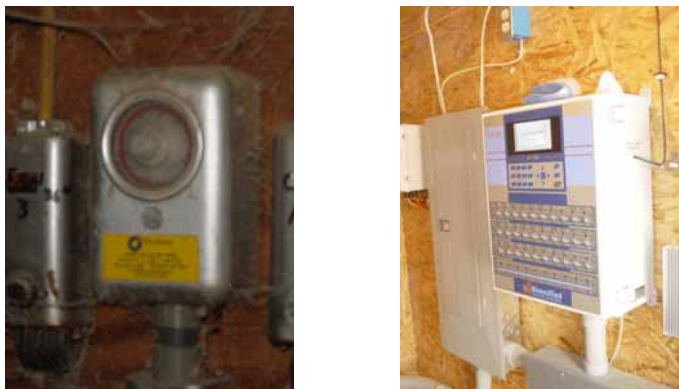
Figure 3. Interval timer or environmental controller to limit pad system cooling.
