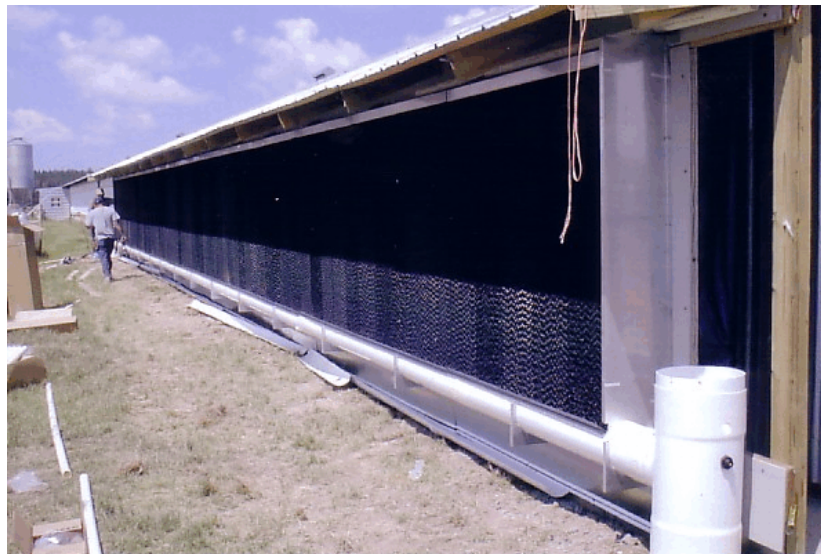
Figure 6. Pad system with a circulation pump on each end.
