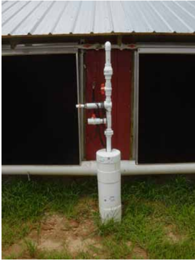
Figure 4. Circulation pump in center of system with cut-off valves
