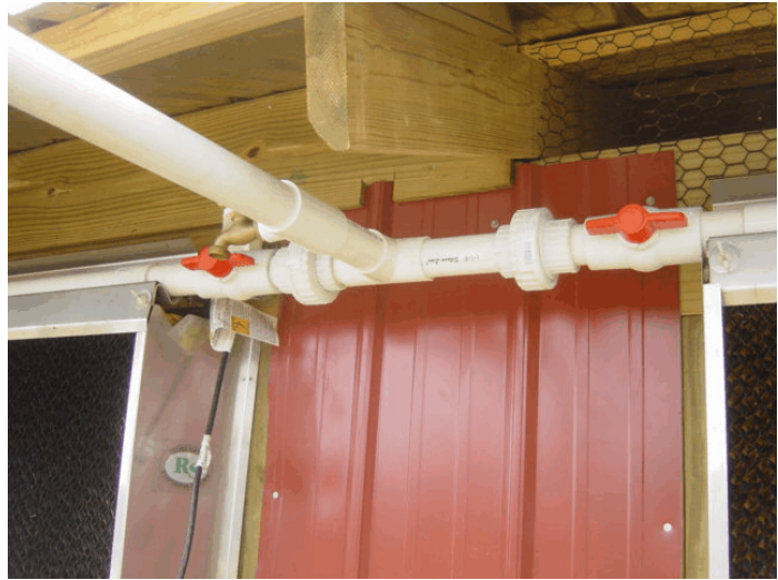
Figure 5. Cut-off valves to control cooling.
