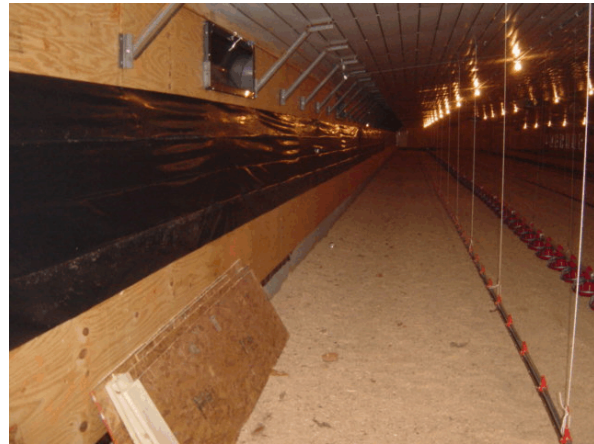
Figure 2. Plastic covering exposed stud wall.
