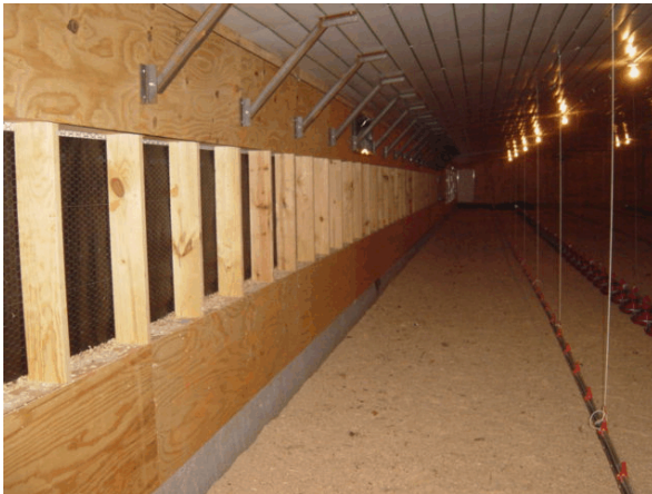
Figure 1. Exposed studs in side wall.
