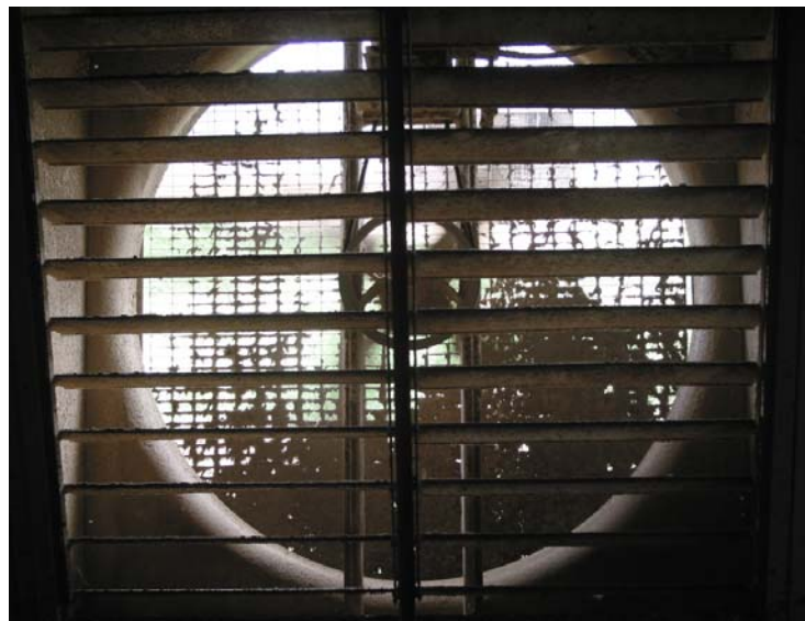
Figure 1. Tunnel fan in need of maintenance.
