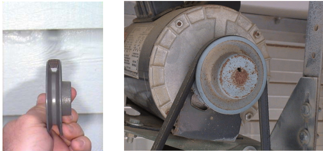
Figure 2. New fan belts
