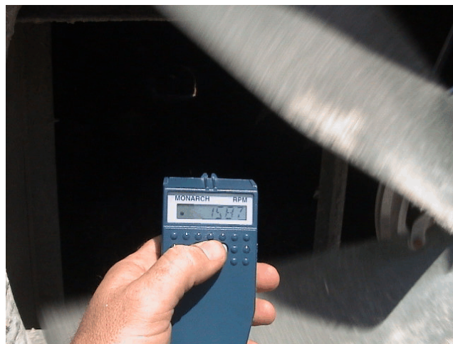
Figure 6. Fan with worn belt.
