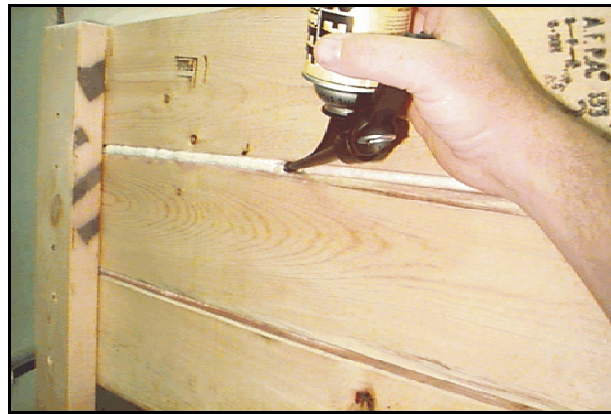
Spray foam insulation filling small crack
