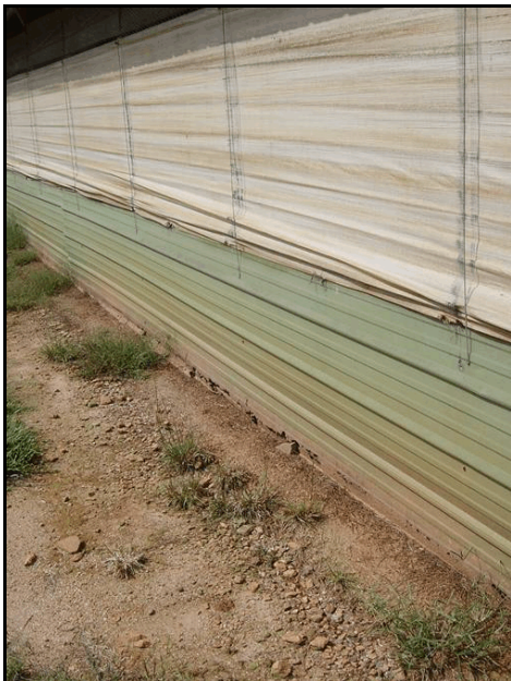
Holes in side wall metal siding
