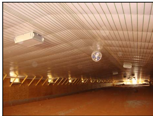
Figure 3. Attic inlets placement in a new 50' wide broiler house
