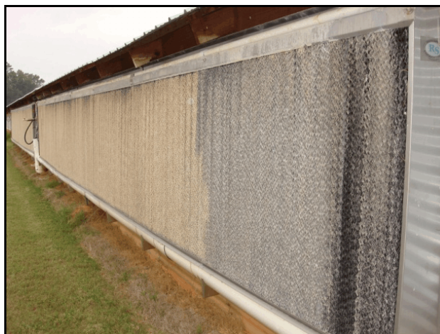
Figure 1. Evaporative cooling pad with mineral build up (partially cleaned)
