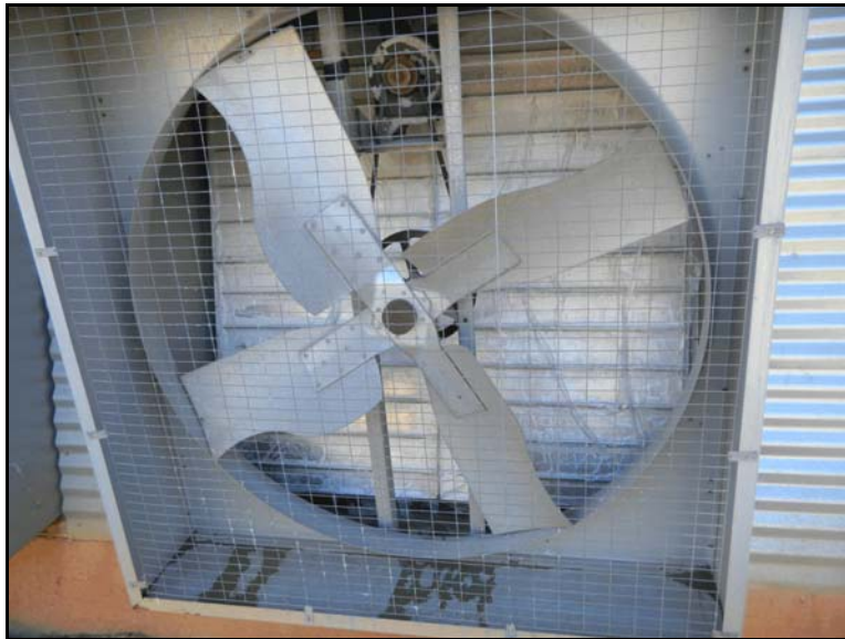
Figure 5. Condensation from covered fan shutter.
