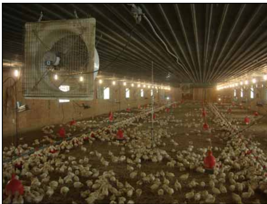
Figure 4. Circulation fan system
