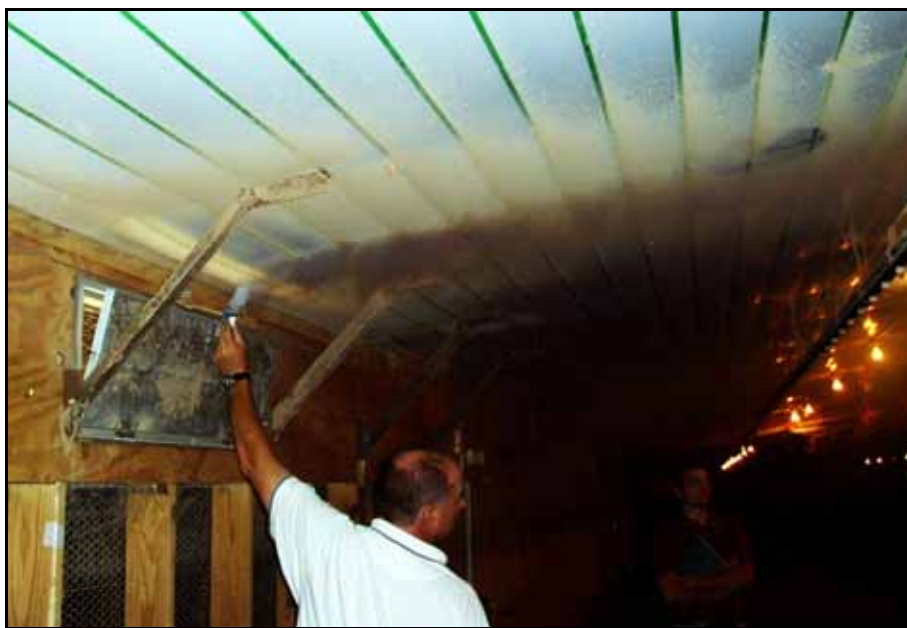
Figure 3. Air flow from a side wall inlet open 2" with a static pressure of 0.10"
