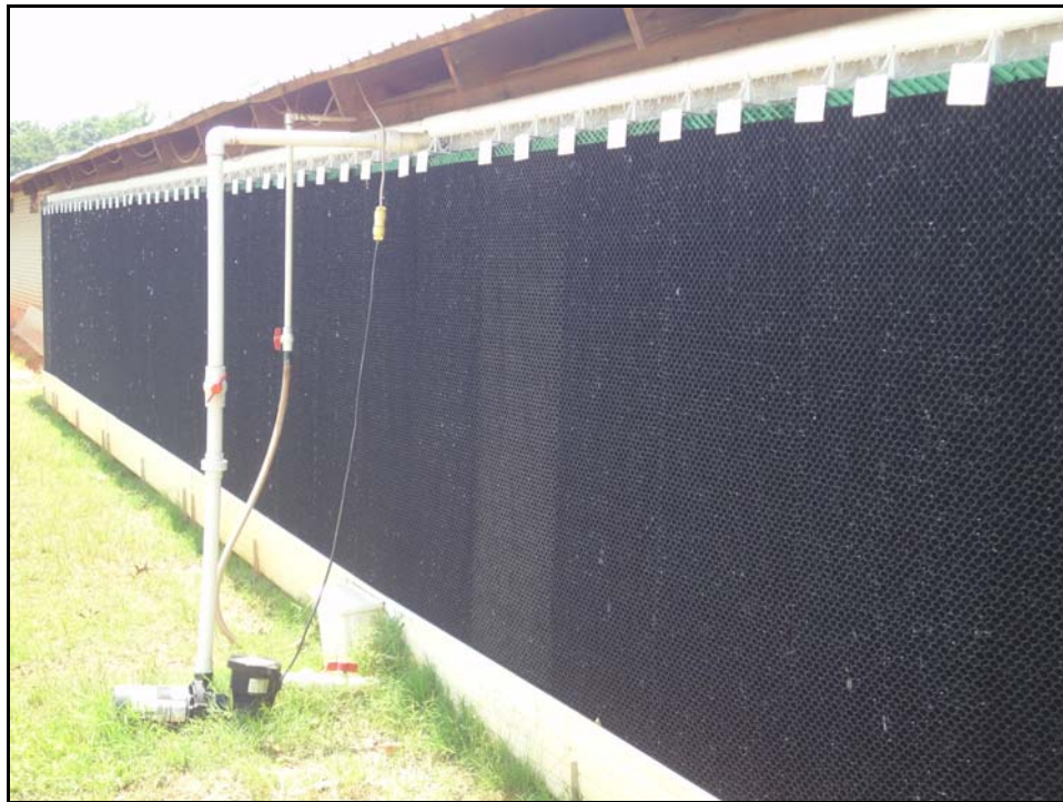
Figure 1. Evaporative cooling system with plastic pads.
