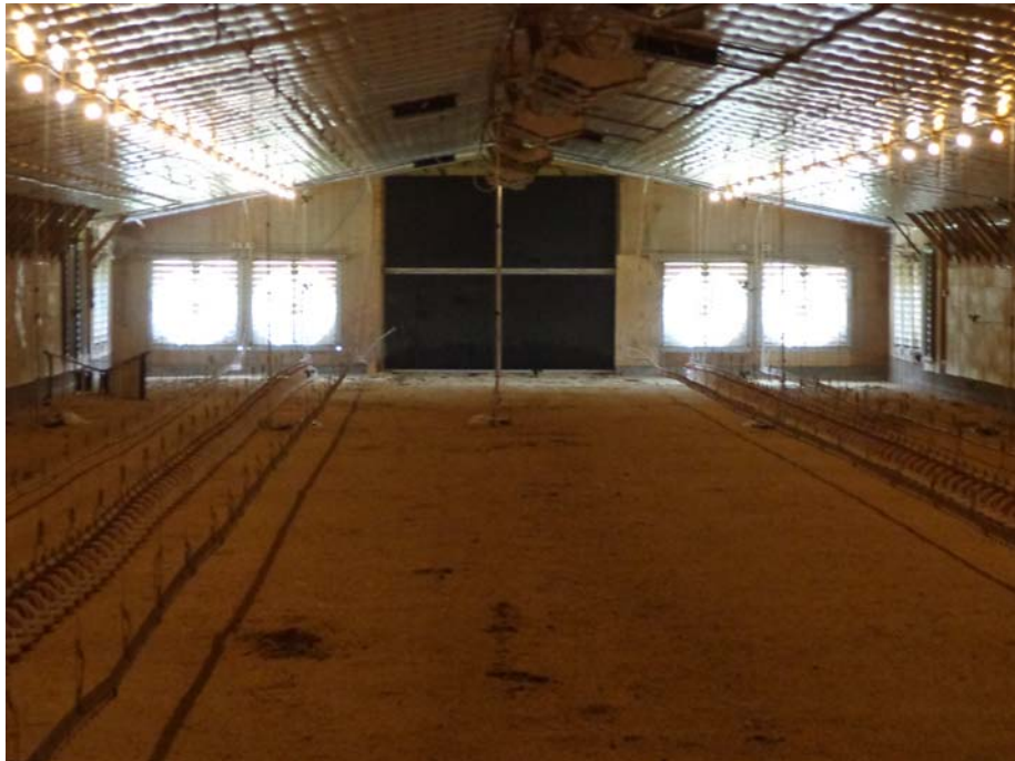
Figure 9. Totally enclose 40' wide house with radiant heaters installed at ceiling peak.
