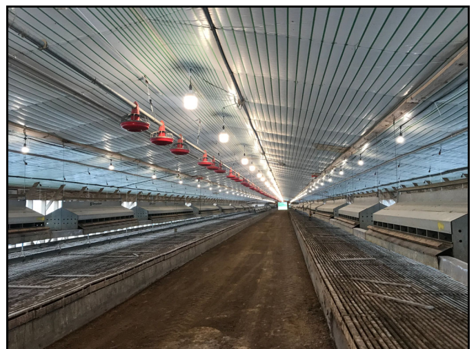
Figure 5. Installed LED lighting system
