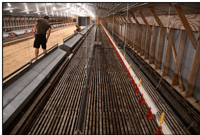
Figure 14. 40-watt HPS lights 20 feet on center with 10-watt LEDs over nests.
