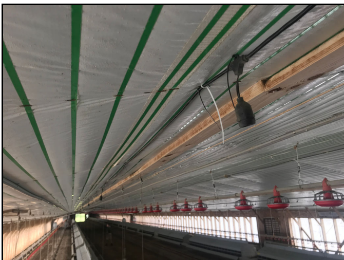
Figure 4. Installed cord set with socket over nests
