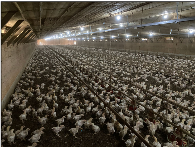
Figure 1. Tunnel fan end
