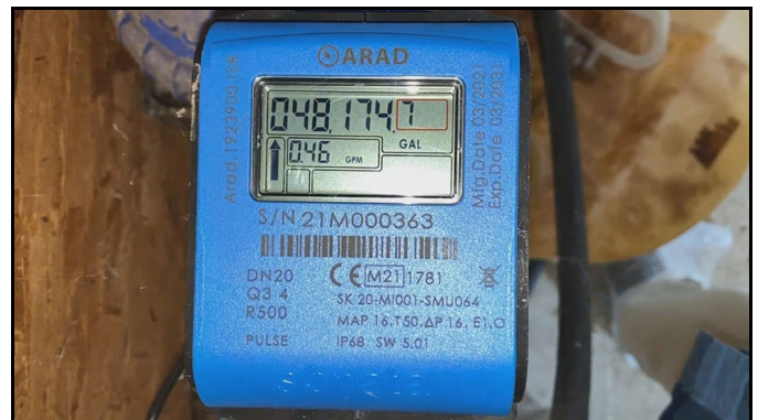
Figure 4. Tunnel fan end water meter
