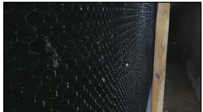
Figure 3. Large water droplets being pulled into the pad room by air flowing through relatively large U-shaped flutes
