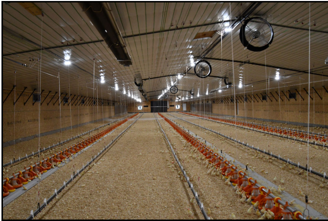
Figure 1. Circulation fan system in a 60' X 600' house
