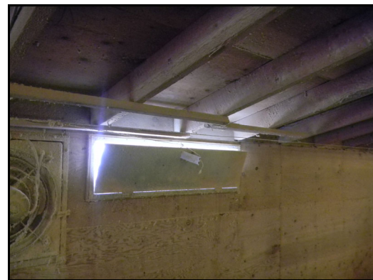
Figure 4. Opening alongside of galvanized inlet opened three inches
