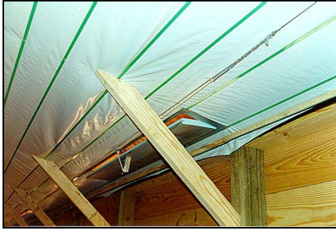
Figure 6a. Ceiling inlet and high tensile wire.
