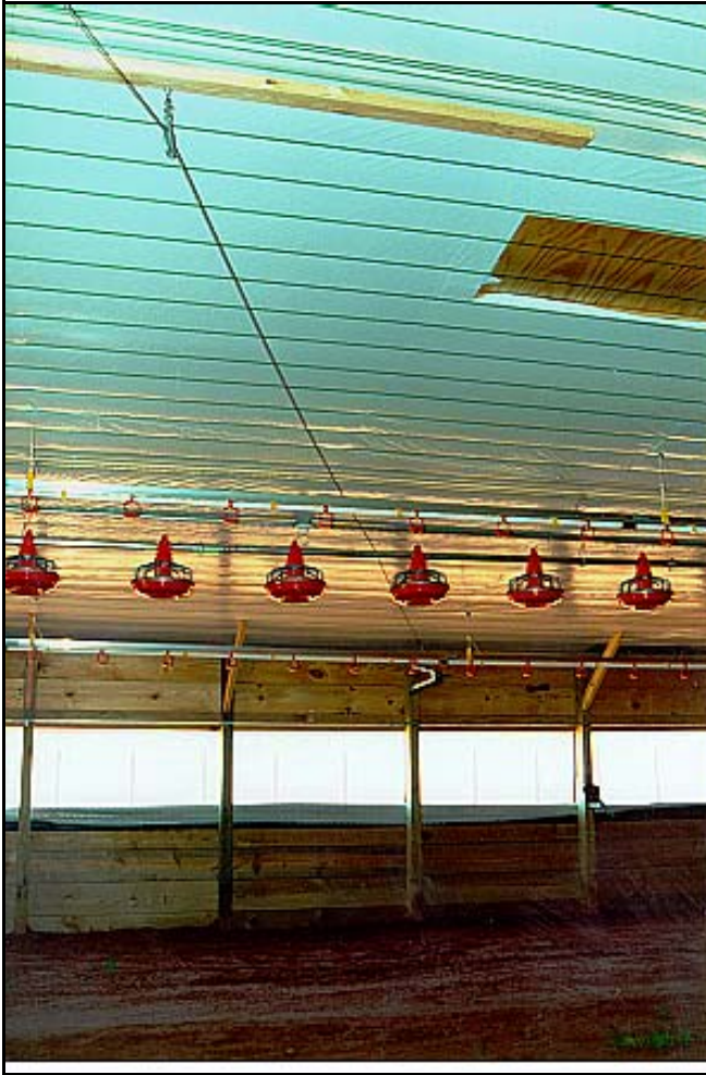
Figure 2. Inlet cable directed across house to inlets on opposite side of house.
