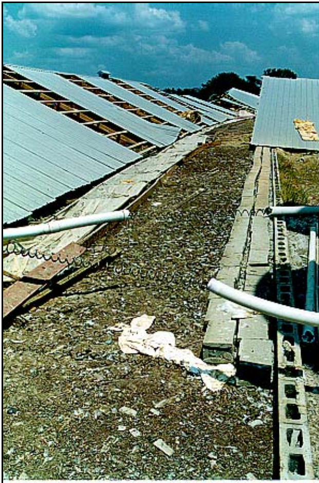
Figure 1. Wind damaged broiler house.
